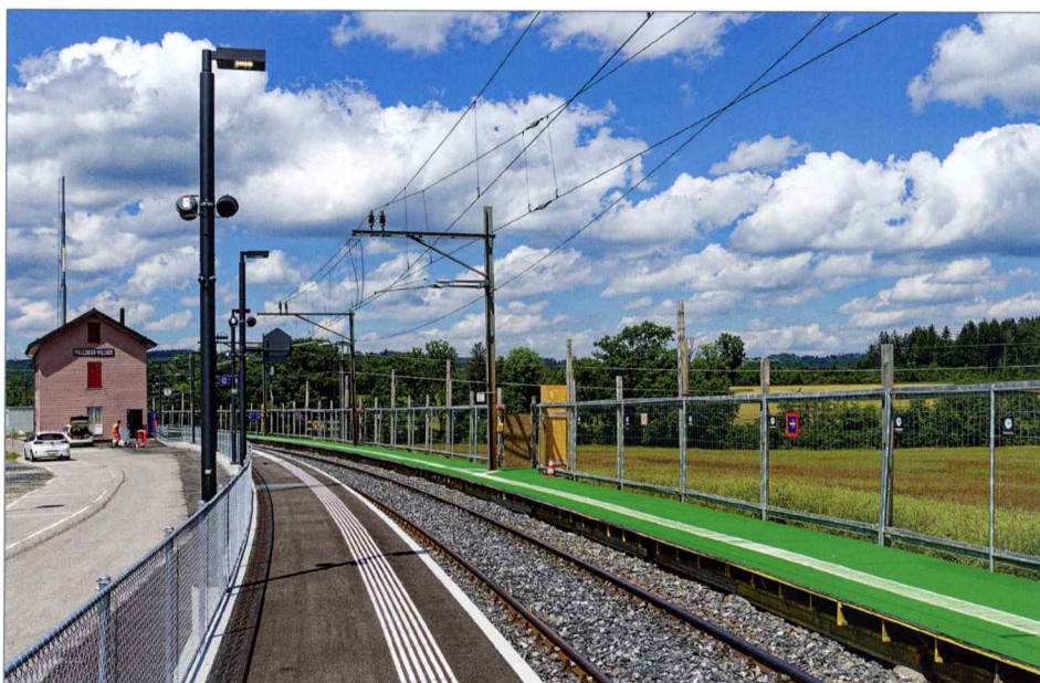
Palézieux-Village station, shortly after completion of the conversion work: On the left, the new platform raised to 55 cm above the top of the rails; on the right, the temporary platform used during the remodelling work, which was about to be dismantled. 13 June 2024.
